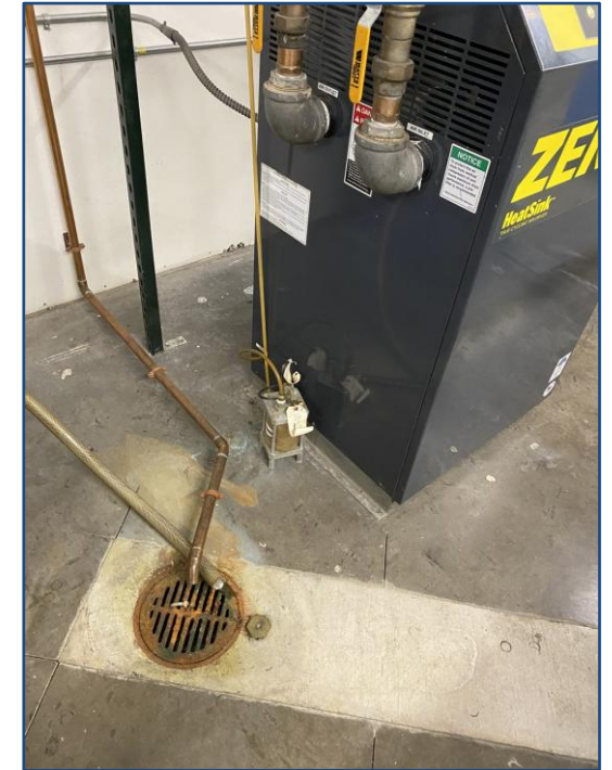
A dryer draining straight to a floor drain — note the oil staining around it
