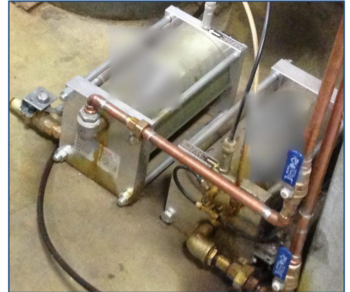
Zero-loss electronic drains on a receiver — note the individual lines & isolation valves — Pneumatic Powered Drains
