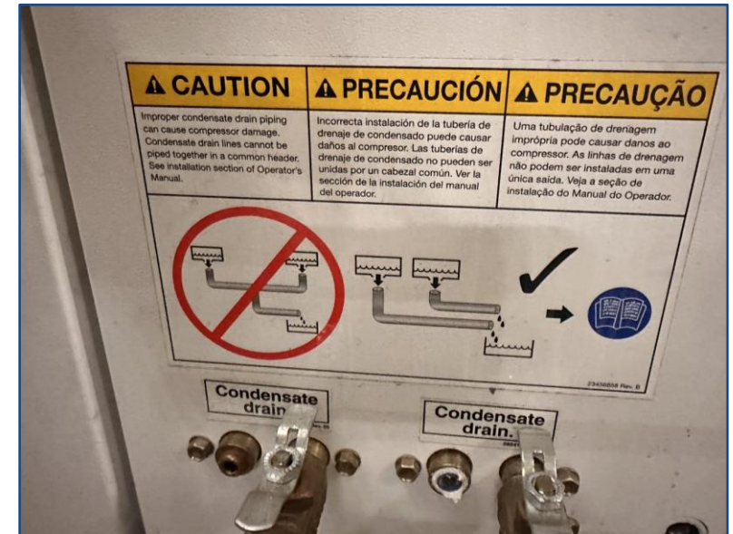
The compressor OEM's own warning: drain lines cannot share a common header
