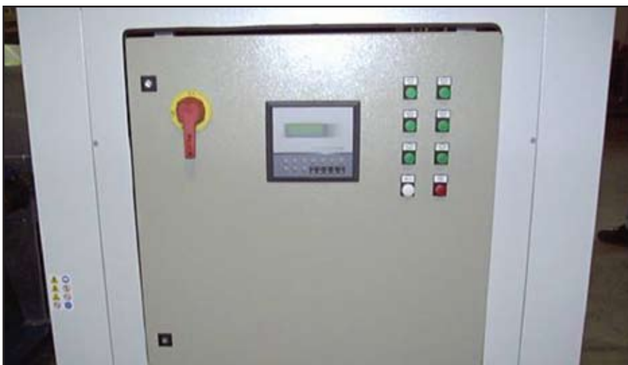
Air Dryer PLC NEMA 4 Control Panel
