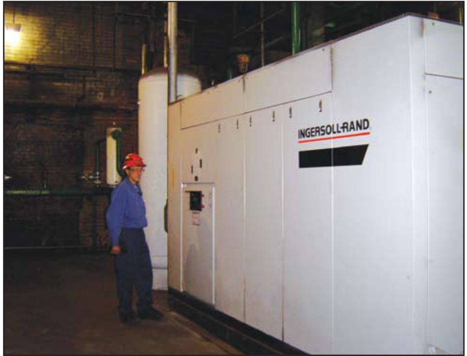
Mr. Richard Deveaney with the 350 horsepower air compressor used in the old centralized plant air system
