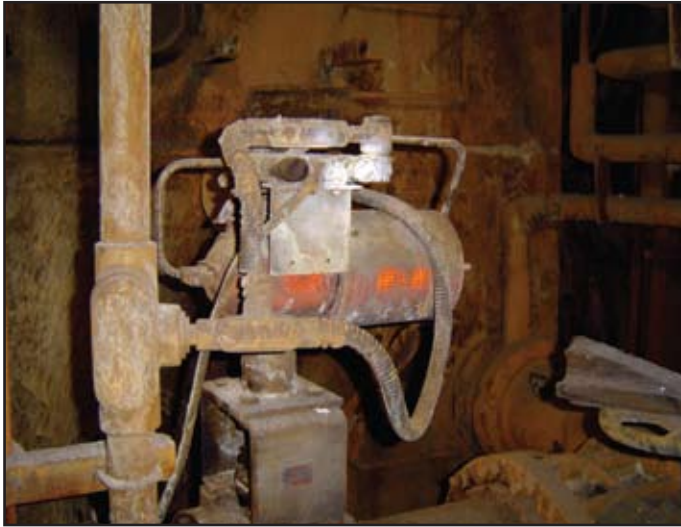
The air-leak audit discovered leaks (painted white) on the Versa-control solenoids used on boilers
