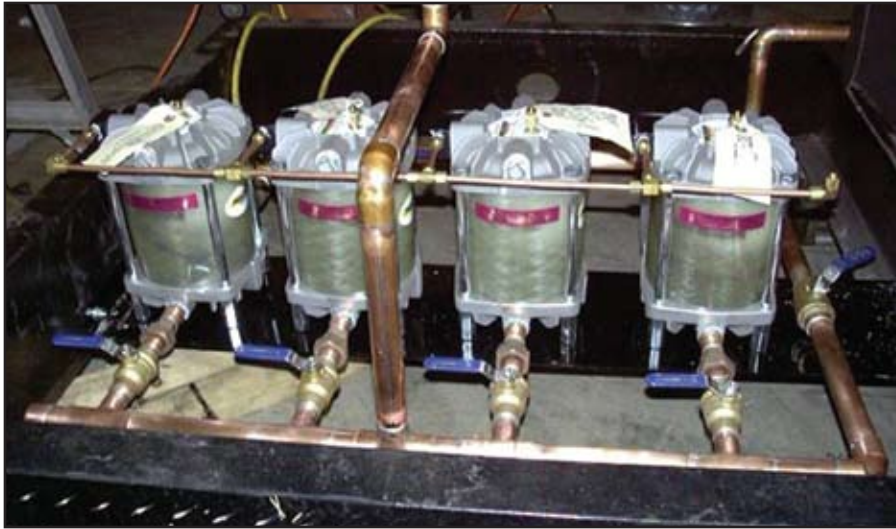
Reliable and Efficient Drain Valves Are Critical
