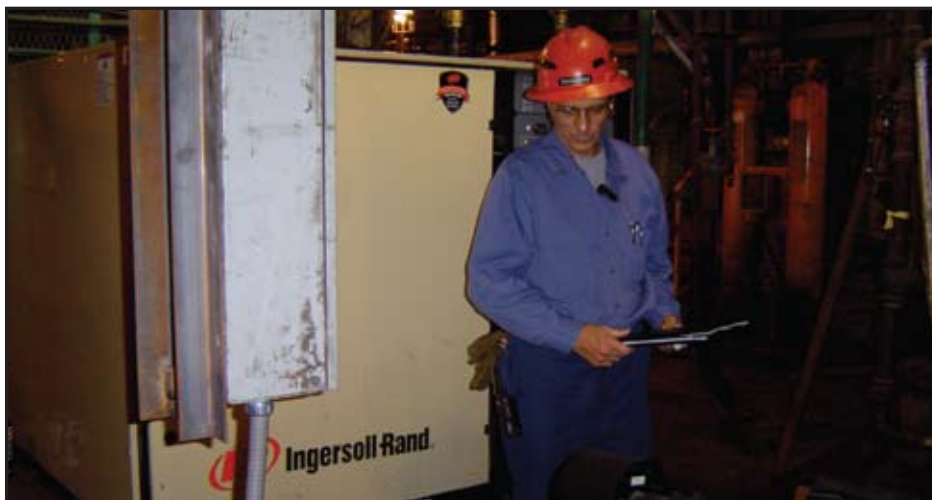
Mr. Richard Deveaney with the 50 horsepower air compressor used for tool air in the new de-centralized plant air system
