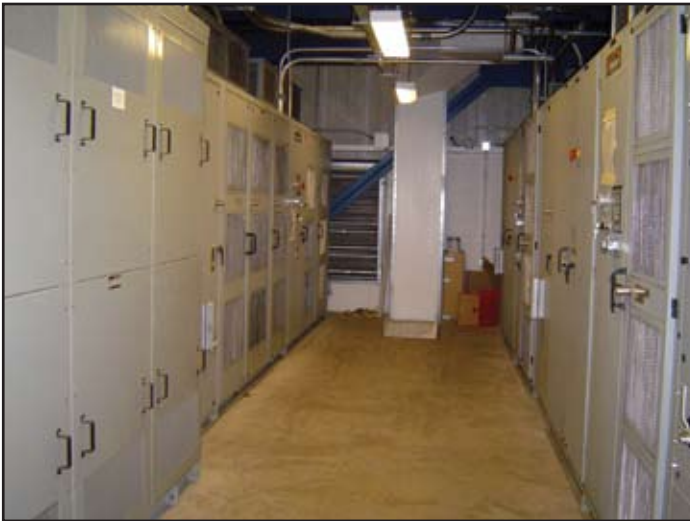
The Transformers Simulate All Power Conditions
