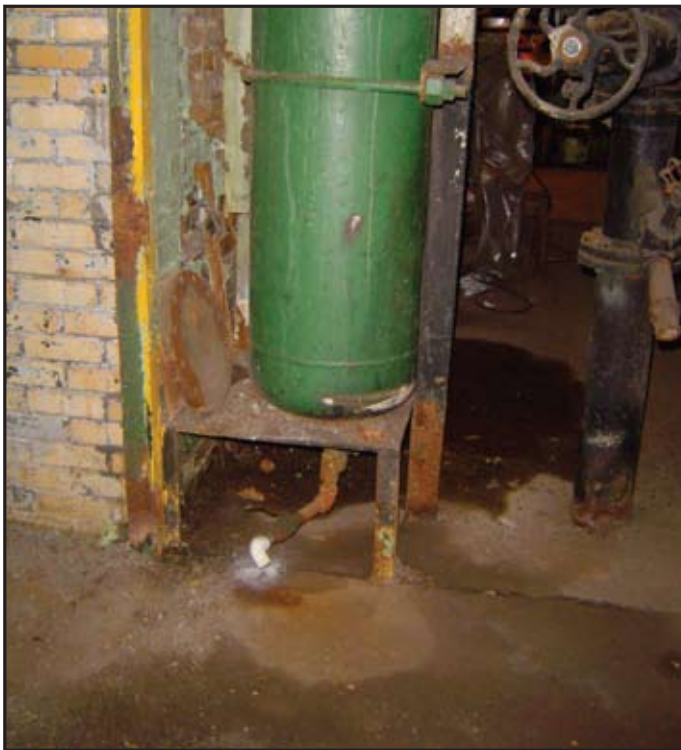
Condensate shut-off valves (painted white) were discovered as air leak locations
