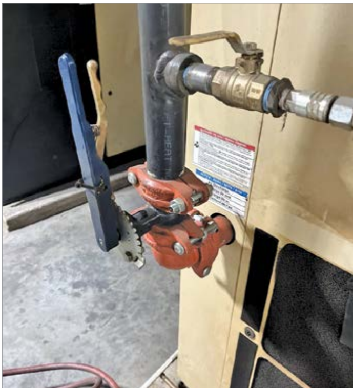
A worn and leaking compressed air system component was identified during routine service. While the condition was not immediately disruptive, it contributed to system instability and highlighted the need for better visibility into long-term operating behavior.
