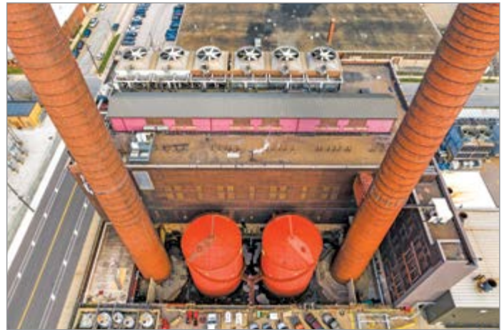
The district energy system runs two three-cell induced-draft crossflow cooling towers located on the roof, and a newer four-cell cooling tower with direct-drive fans and variable-frequency drives in a parking area.
