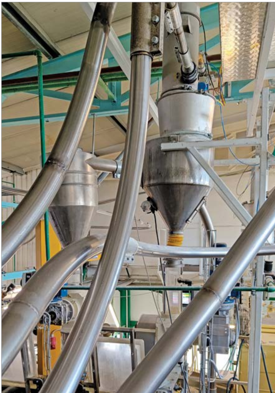
A flour conveyor in Wolf Nudeln's manufacturing facility. (Source: Busch Group)
