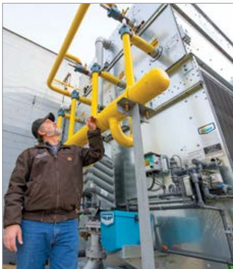
Technicians inspect a critical process evaporative condenser at a cold storage facility, equipped with a factory-mounted solid water treatment system designed to provide streamlined water treatment control, improved system cleanliness and optimized equipment operation.
