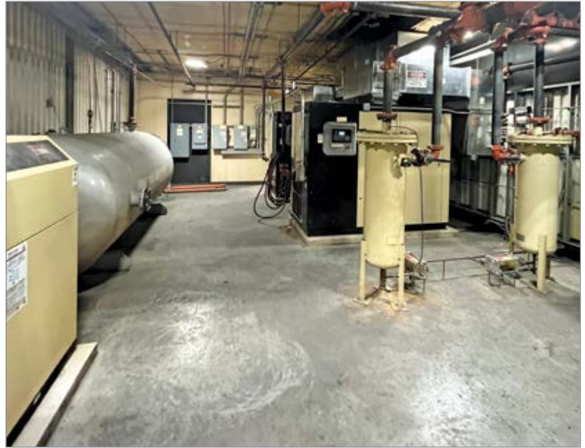
The facility's oil-flooded rotary screw air compressors discharge 100-125 psig (6.9 to 8.6 barg) compressed air to a horizontal wet receiver tank, with downstream compressed air dryers, filters and overhead piping supplying plant air for CNC laser cutting, powder coating and assembly operations.
