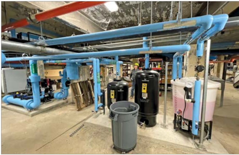
A glycol fill station, expansion tanks and piping equipment in the basement
