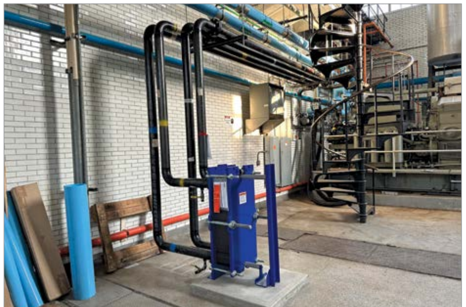
The diesel pump engine heat exchanger
