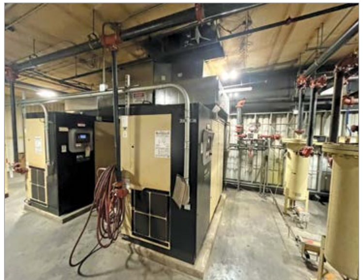
The facility's compressed air system includes dual oil-flooded rotary screw air compressors, along with compressed air dryers and coalescing filters, configured so one system operates while the second remains available as backup.
