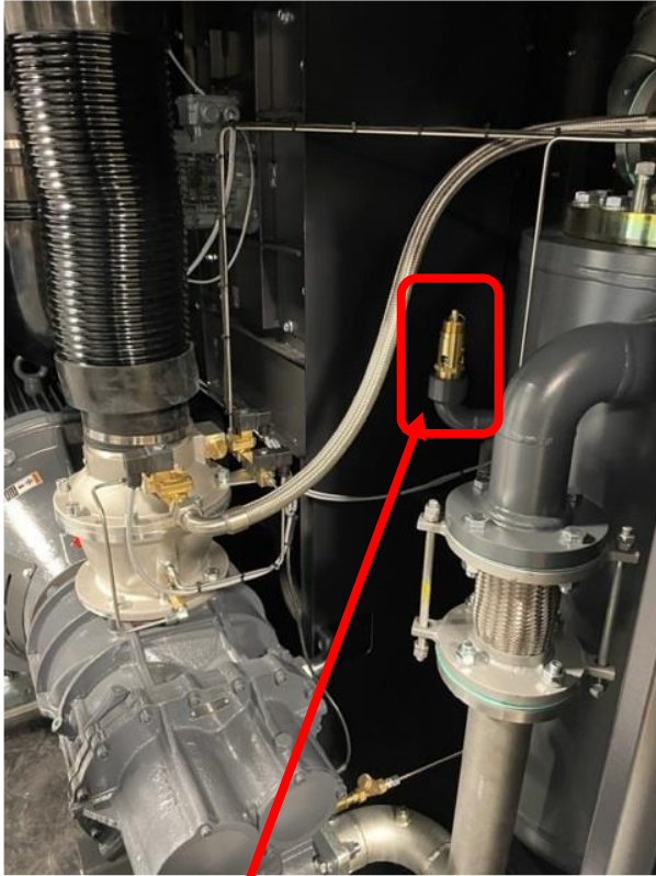
❖ Tank Safety Relief Valve
