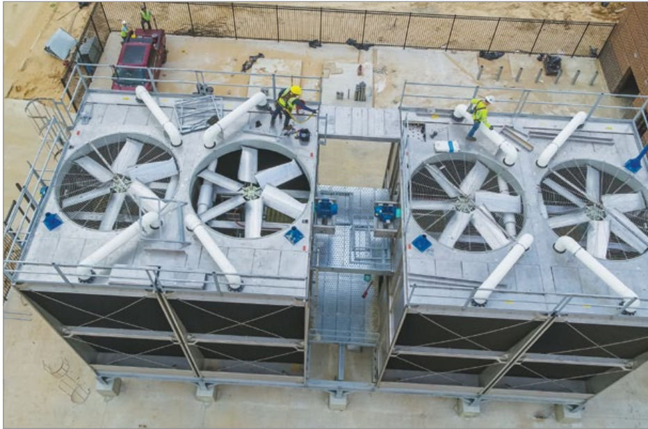
S&S HVAC team members providing "trim out" work installing a SPX Marley cooling tower at a Houston area high school.
