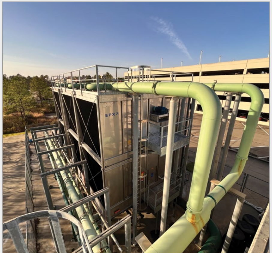
S&S HVAC worked closely with a mechanical contractor to reconfigure cooling tower piping.
