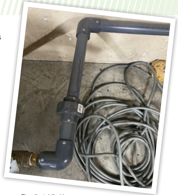
The client drilled in screws to secure fittings and elbows in plastic PVC piping being used for the compressed air system. This is at risk to explode and harm workers. Photo credit: Daniel Smayda, Advance Air Compressor Sales & Repairs
