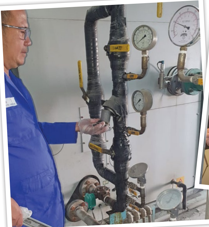
↑ In Saudi Arabia, reader Melchor Operiano services a Wye strainer to keep cooling water free from obstruction. Melchor is an environment and sustainability coordinator for Middle East Battery Company. Visit https://mebco.com
